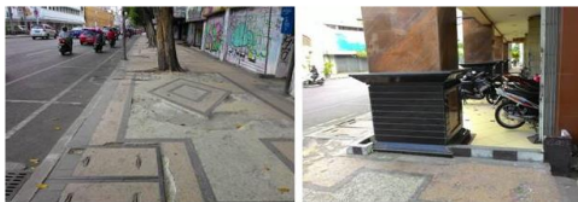
Figure 9. Pedestrian ways are damage and vehicles parking on the pedestrian
